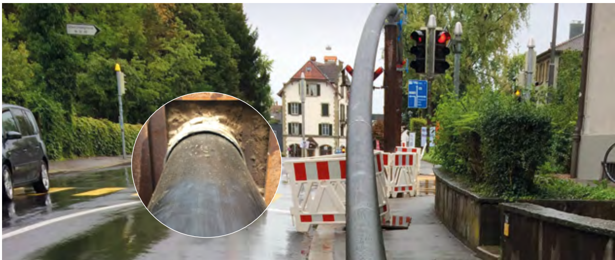
The pre-welded SIMONA® PE 100 liner pipe is drawn through a tapered die, thus reducing the cross-section. Due to the elasticity of the material, the pipeline expands again and provides a snug fit round the inside wall of the old pipe.
